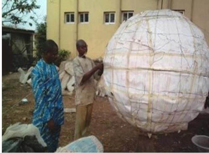
Plate 9: Globe Armature Covered with White Cardboard Sheets © The researcher, 2018
