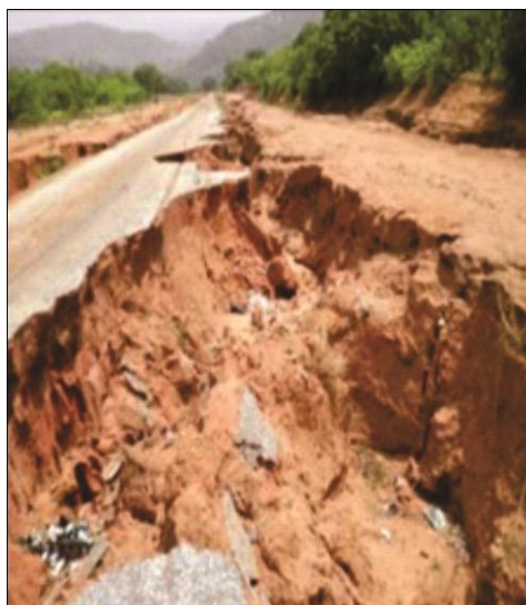
Plate 1: Amuda-Achara Isuochi Road Gully Erosion
