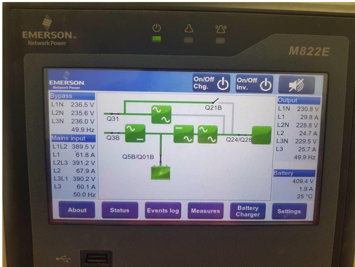
Figure 4 UPS Control screen
