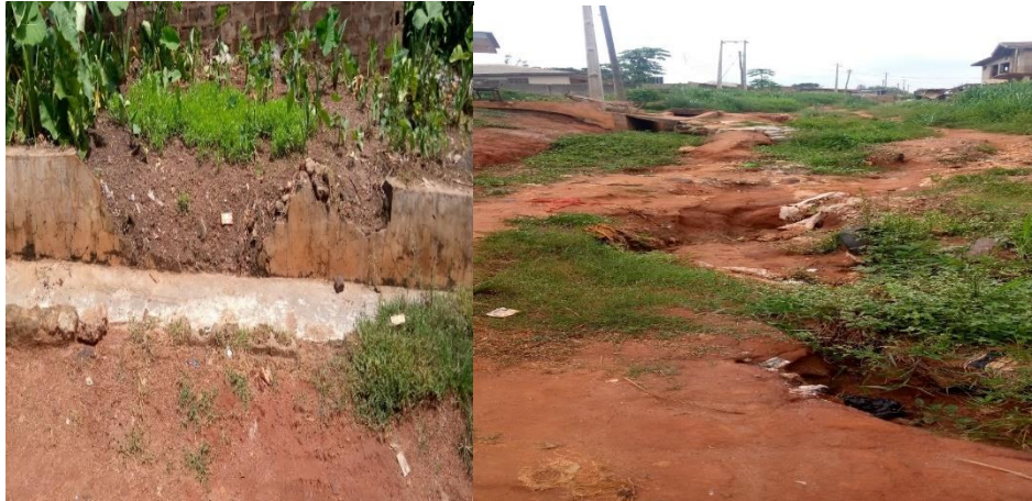
Plate 8: Damaged existing drainage
