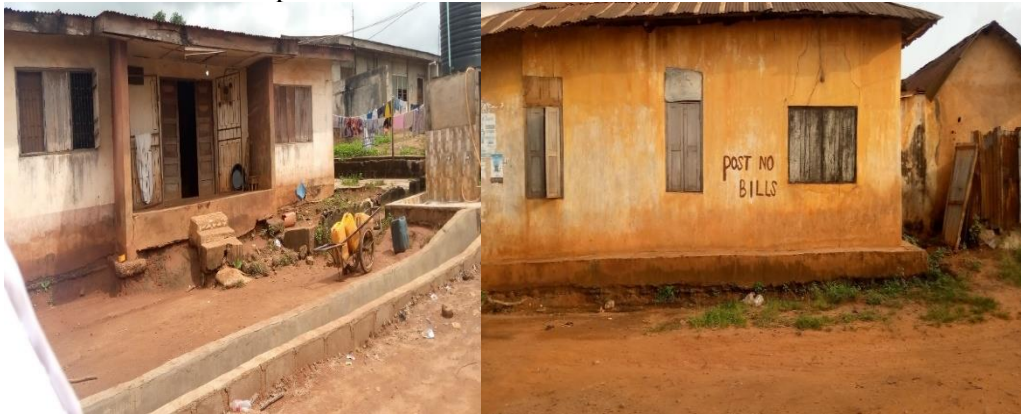
Plate 4: A residential building with an exposed foundation
