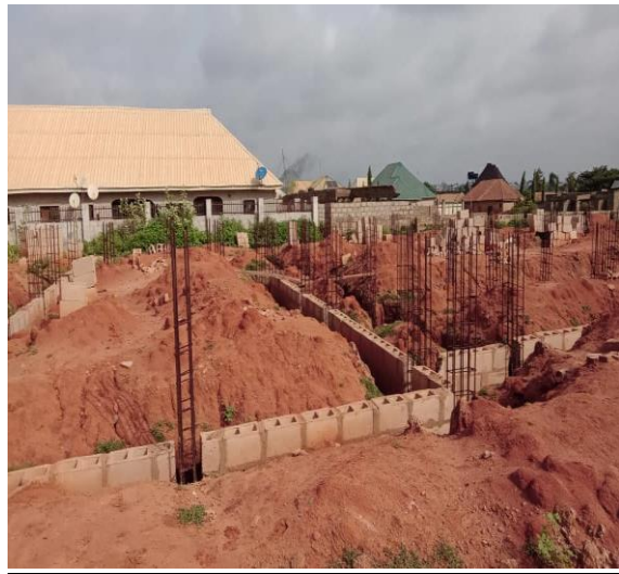
Fig 6: Ongoing construction of the temporary site of proposed IMAN University of Medical Sciences, Bida
